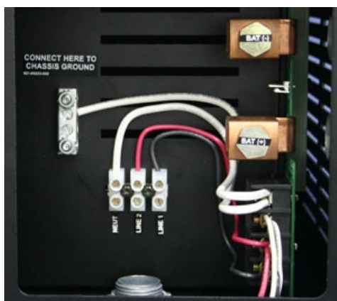
4KW BI-PHASE SYSTEM
